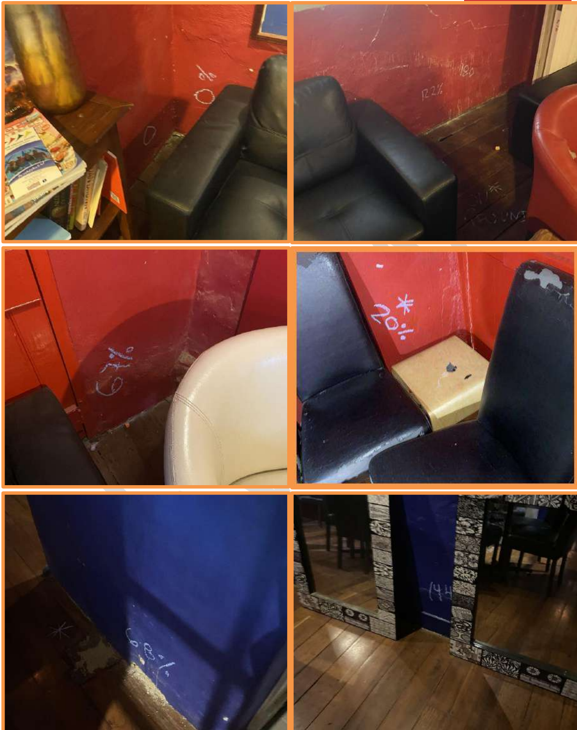
Figure 2q_1: - Moisture Content within Brick Wall Locations Around Rear Restaurant Area
