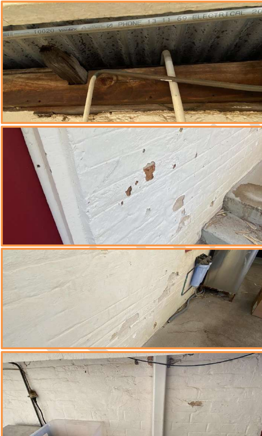
Figure 2g: - Moisture Ingress to wall and timber
