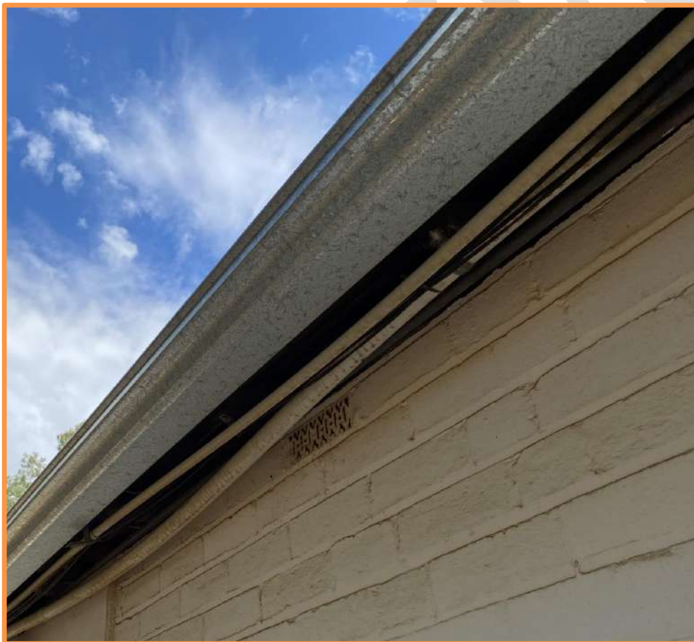
Figure 2c: - Open Gutter and Eaves to Property
