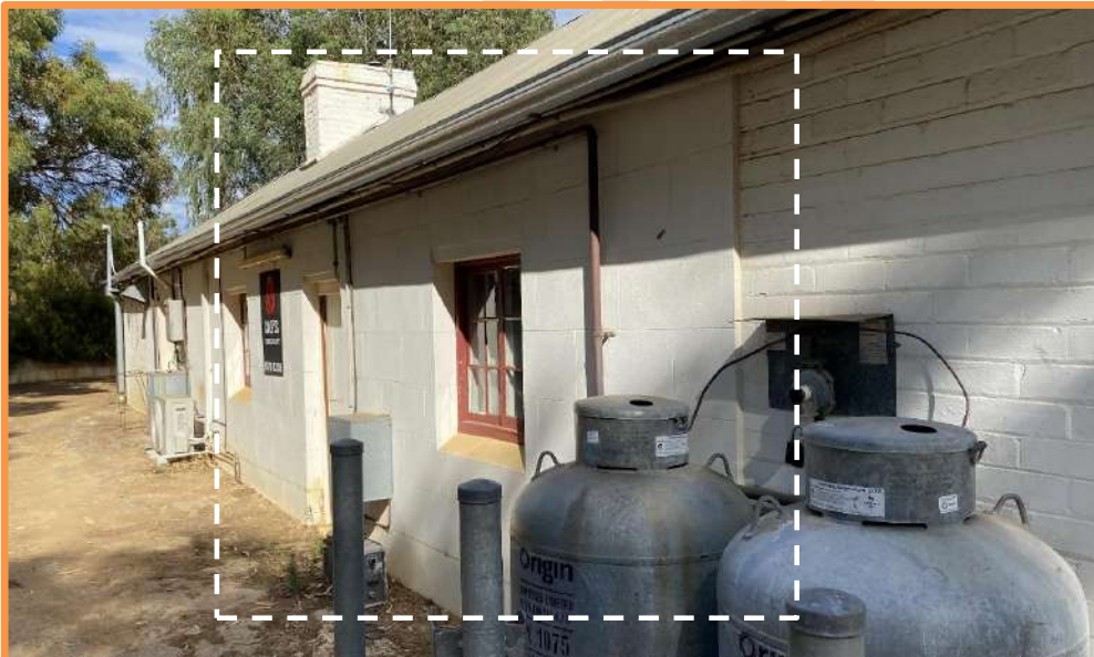
Figure 2b: - Elevation showing Rising Damp
