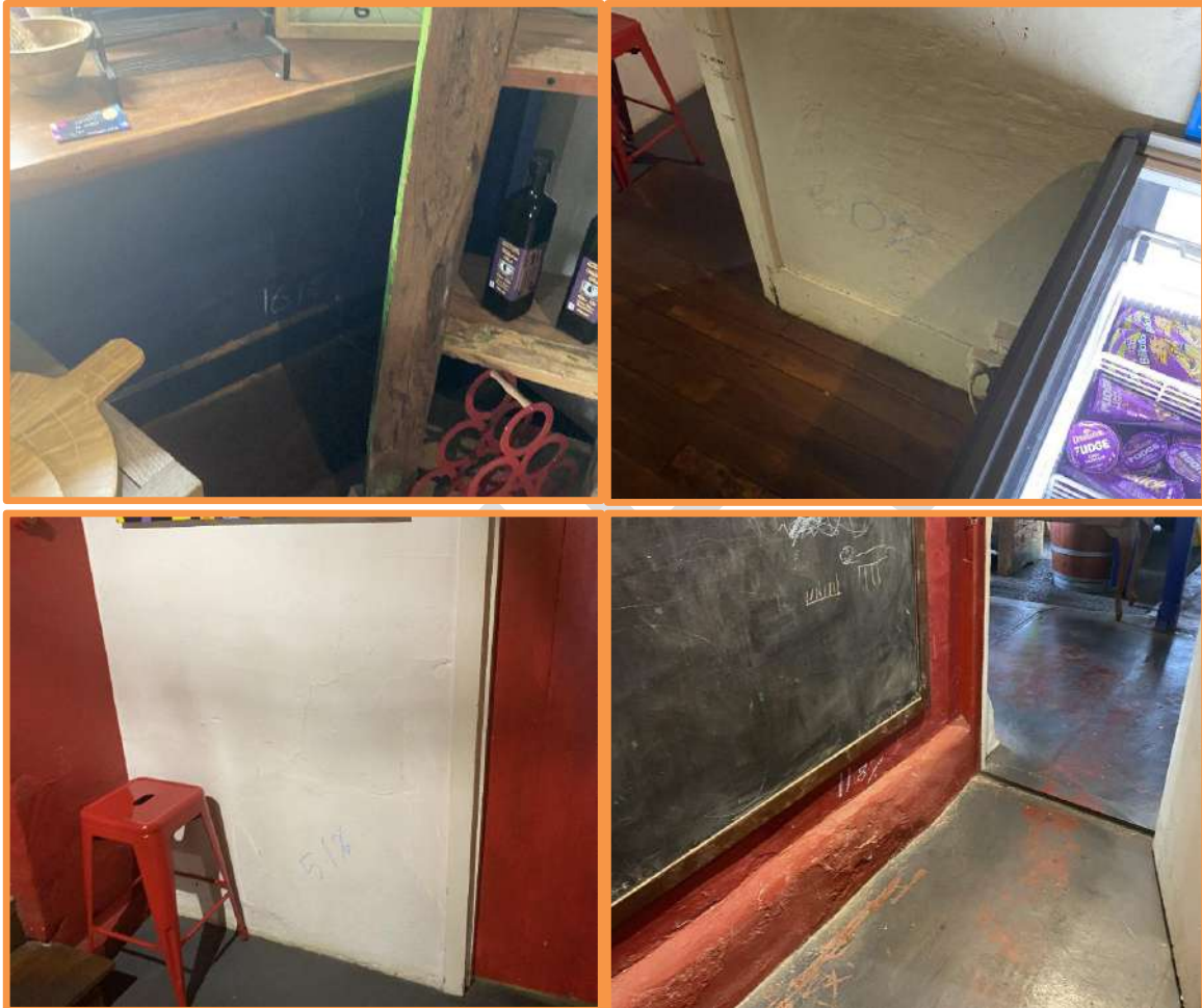
Figure 2p_2: - Moisture Content within Brick Wall Locations around shop/children's area
