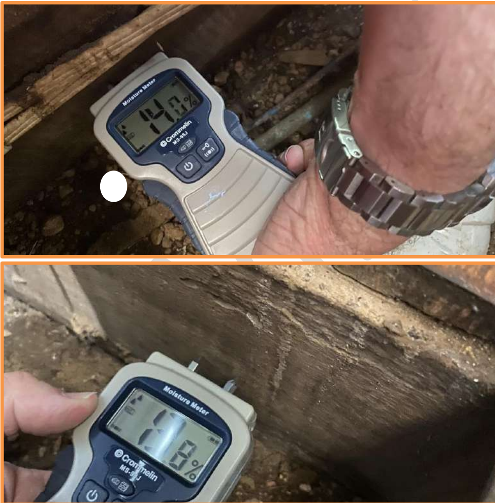
Figure 2m_1: - Moisture Readings on Timber #1;
