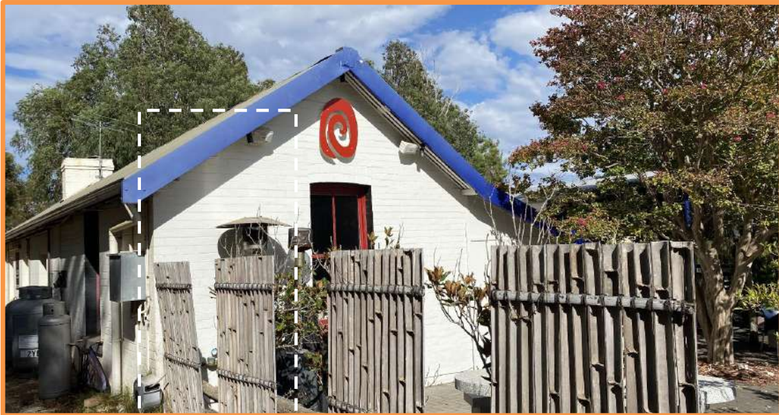
Figure 2a: - Elevation showing rising damp
