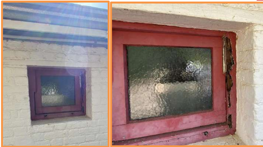
Figure 2f: - Evidence of termite Damage
