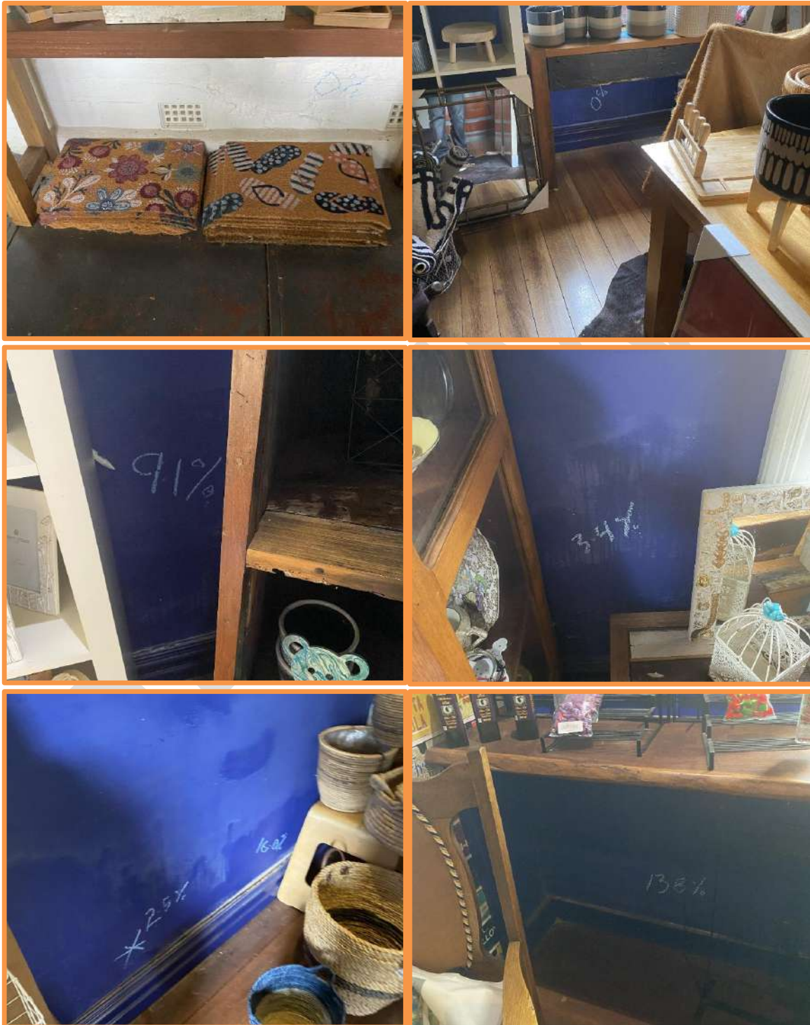
Figure 2p_1: - Moisture Content within Brick Wall Locations around the shop area
