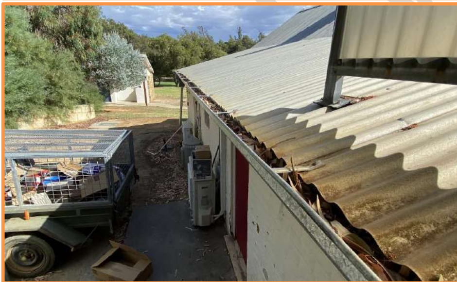
Figure 2h – Clean Gutter of leaf debris
